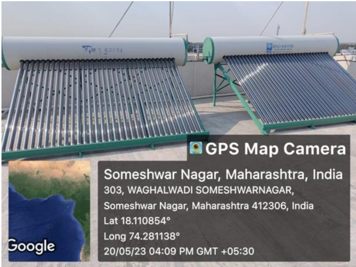
Solar Panel over Girls Hostel
