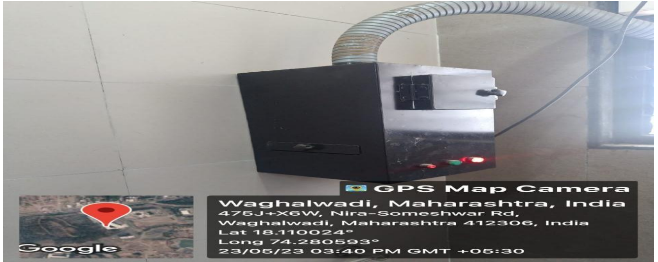
Sanitary Napkin Incinerator At ground floor Ladies Washroom
